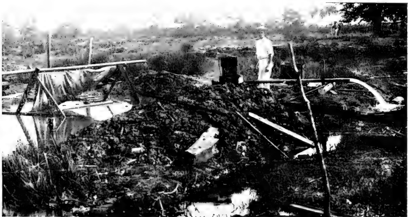
The centrifugal pump in action. The canvas covers the center of the spring. It was impossible to work in the combined heat of the midday sun and hot water without shelter
